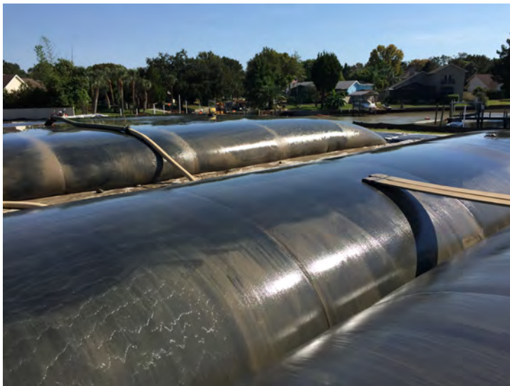
The Triflo Mechanical Dewatering System separates the sediments, while fine mesh filters remove and clean the water, which is returned to the canal.
